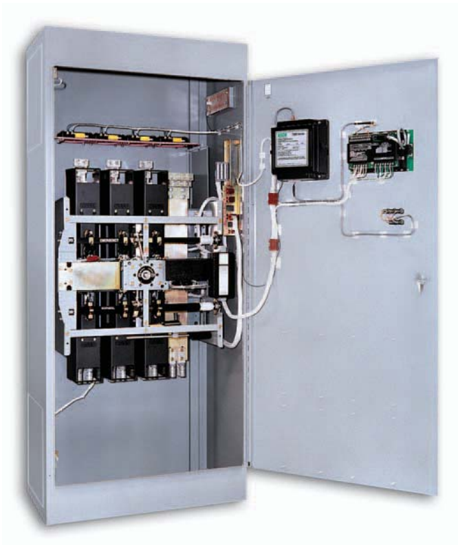
Fig. 1: Three Pole 7000 SERIES Automatic Transfer Switch rated 1600 amperes (shown with optional front connected terminals and Power Manager).
