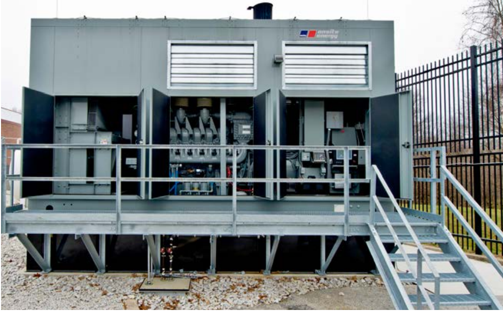
Outside the Cerner Technology Center, MTU Onsite Energy Series 4000 generator sets are contained in Level 2 sound attenuated enclosures.
